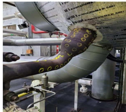
Figure 1: Piping section showing the environment and situation of pipe inspection at Angra nuclear power plant 1. Circles show positions indicated by the engineering group for pipe thickness inspection.
